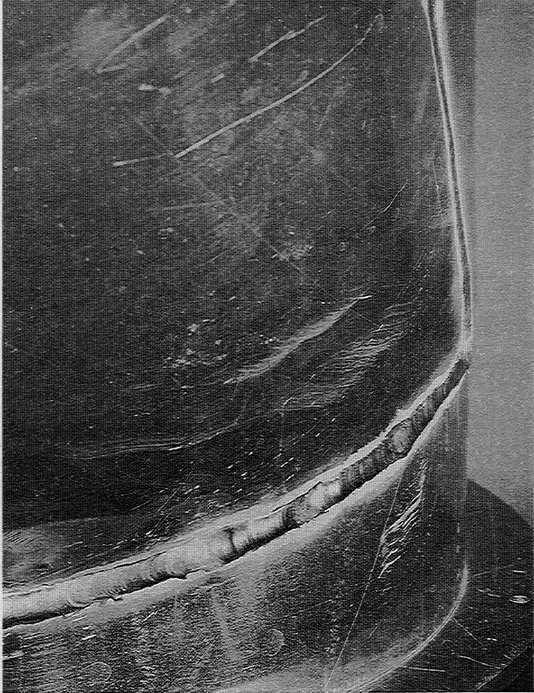
Fig. 3. Closeup of the Irregularity in the Weld at the Intersection of the Members of the 30^{\circ} Lateral.
